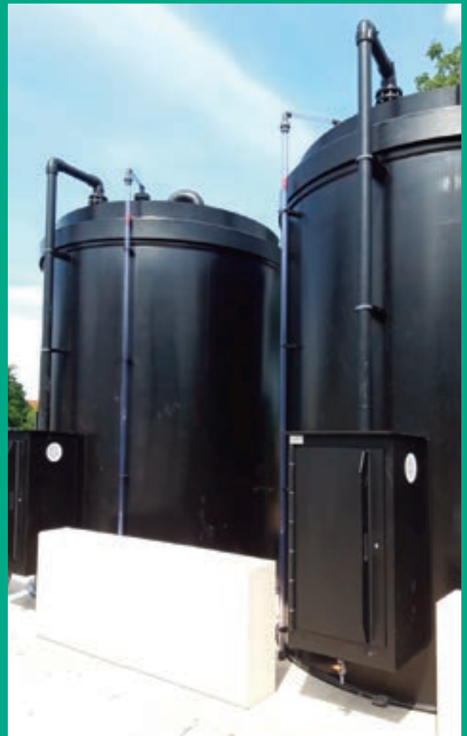
storage tank with filling station
